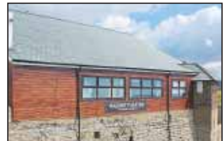
■ WATER TIGHT: The new roof at the Marine Theatre is now completed
